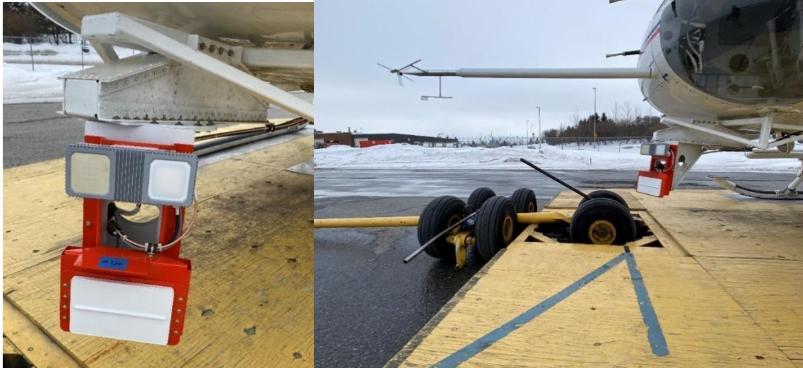
Figure 21: Echodyne (lower) and Fortem (upper) Physical Installation
